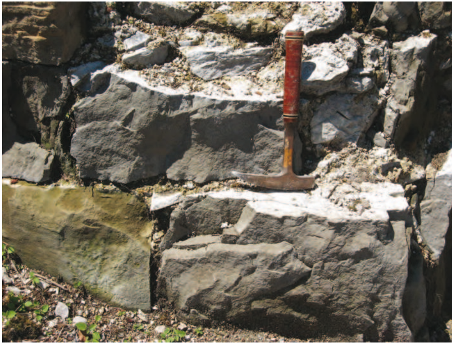
Slika 9.14: Klesani bloki oligocenskega peščenjaka v temelju notranjega obzidja. Taki bloki se v stolpu ne pojavljajo. Na preperavanje je ta peščenjak bolj občutljiv, hkrati pa se ga lahko zelo lepo kleše. Iz tega peščenjaka sta narejena tudi podstavka na dvorišču. Figure 9.14: Chiselled blocks of Oligocene sandstone in the foundation of the inner wall. Such blocks were not found in the tower. While easy to chisel, this type of sandstone is prone to weathering. The two pedestals in the courtyard are made from the same sandstone.
