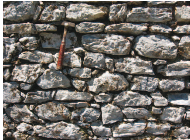
Slika 9.16: Zunanje obzidje. V njem so urejeno zloženi lomljeni plastnatega apnenca z vrba Starega gradu. Osnova za malto je savski prodnat pesek.. Figure 9.16: Outer wall. It was made of well chiseled limestone blocks. Mortar was here made of lime and gravelly sand from the Sava river.
