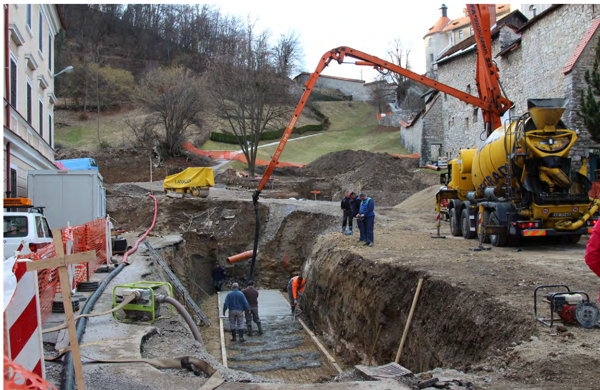
Slika/ Figure 11 Pogled na gradbišče pri urejanju Trga pod Gradom in otroškega igrišča (foto J. Štukl). / A view of the construction site during renovation of Trg pod Gradom and the construction of a children's playground (photo by J. Štukl).
