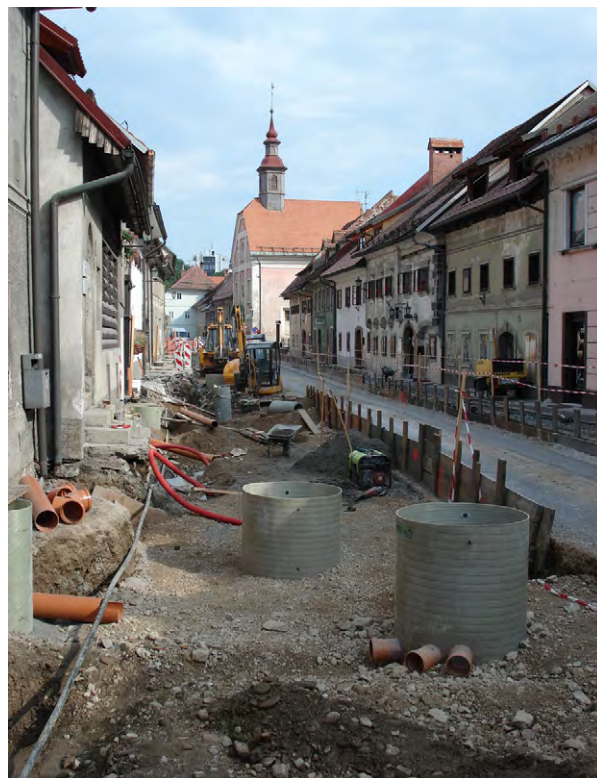
Slika/ Figure 5 Pogled na Spodnji trg med sanacijo vodovoda in arheološkim dokumentiranjem ob gradnji (foto J. Štukl). / A view of Spodnji trg during renovation of the water supply system and the archaeological watching brief (photo by J. Štukl).
